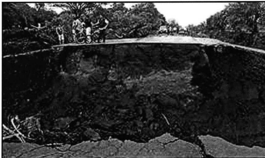
Figure 11.0 – Mitch Caused Massive Road Damage, Honduras
